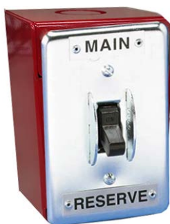
Figure 20. Main and Reserve Transfer Switch
